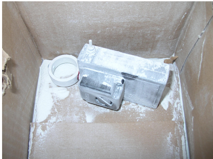
Figure 3. As seen in the picture, the unit was well covered with powder, and the surrounding box is still in tact.
